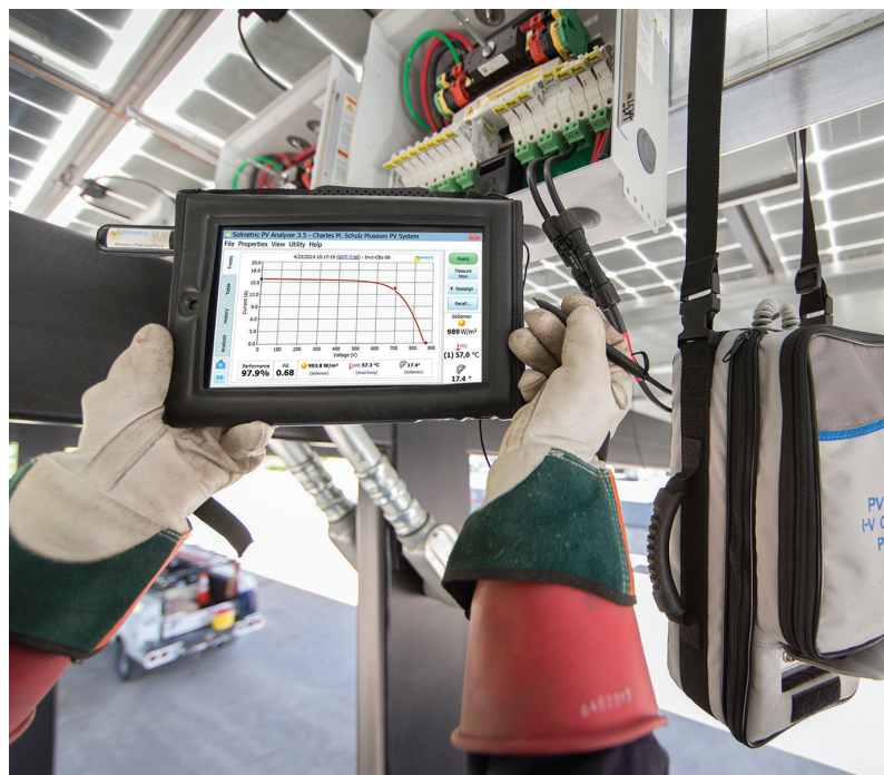
Figure 2 This I-V curve trace has a normal shape and a performance factor greater than 90%, which indicates that the test circuit is performing as expected. In this case, the technician will save the data and test the next circuit.
